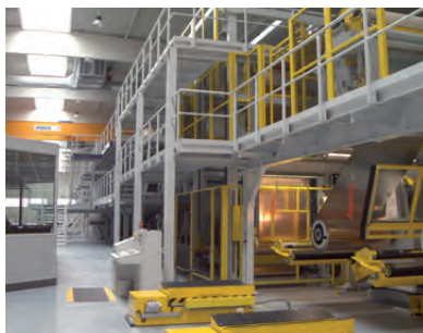
PVD technology vega plant
